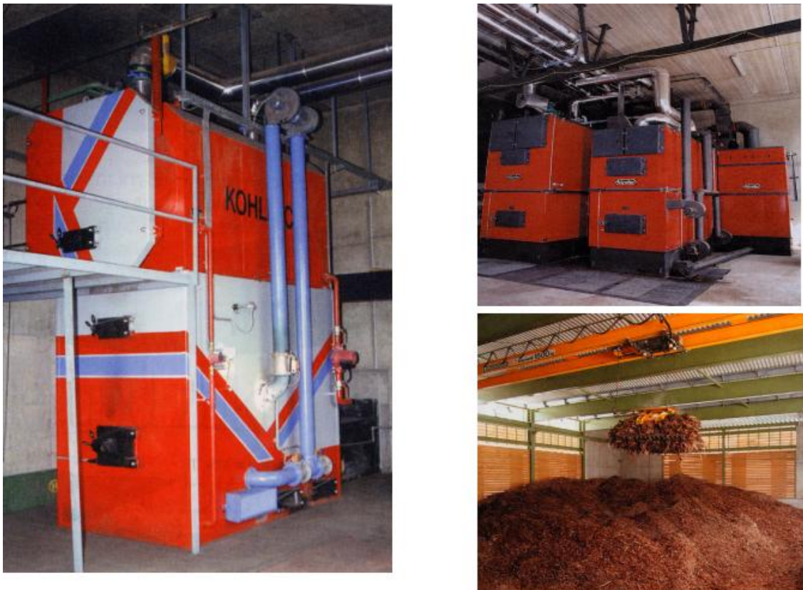
Fig. 14b: Biomass boilers for district heating
