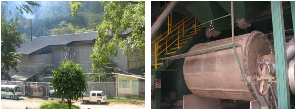
Fig. 3: Coffee drying, Coopeldos, Costa Rica, Installed capacity: 595 kW th (850 m 2 Solar Wall collector)
