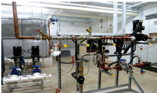
UWCSEA's hot water system
