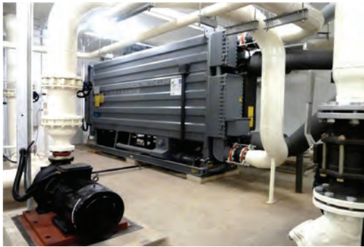
UWCSEA's adsorption chiller
