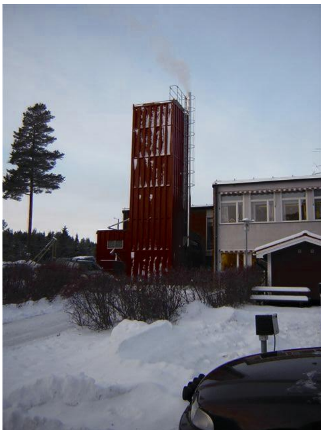
Increase the use of biofuels in middle-scale heating plants (50 kW . 1 MW)
