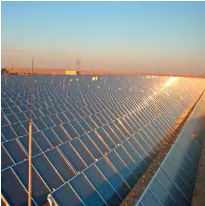
36.300 m 2 Anlage in Riad, Saudi-Arabien, Foto: Millennium Energy Industries
