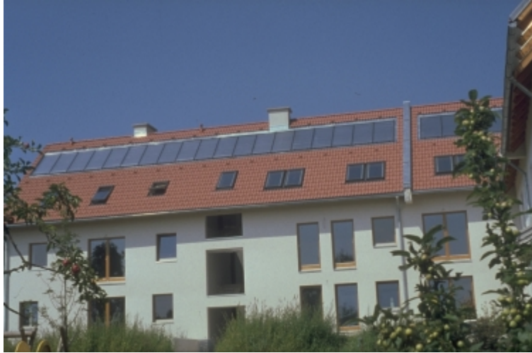
Figure 16a. Hot water preparation in a multi family house
