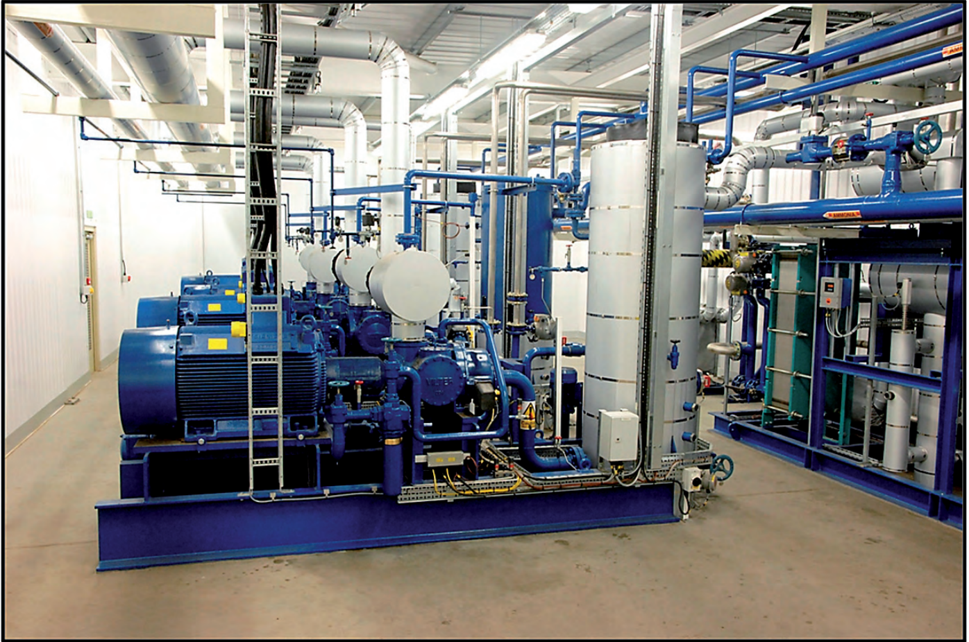
Figure 5 Self-contained ammonia heat pump for food processing
