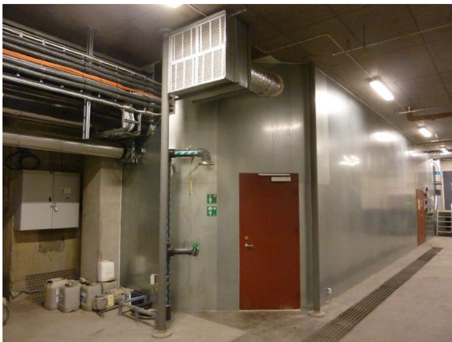
Figure 4. Gas-tight machinery room with separate ventilation system [Photo: Eptec Energi AS]
