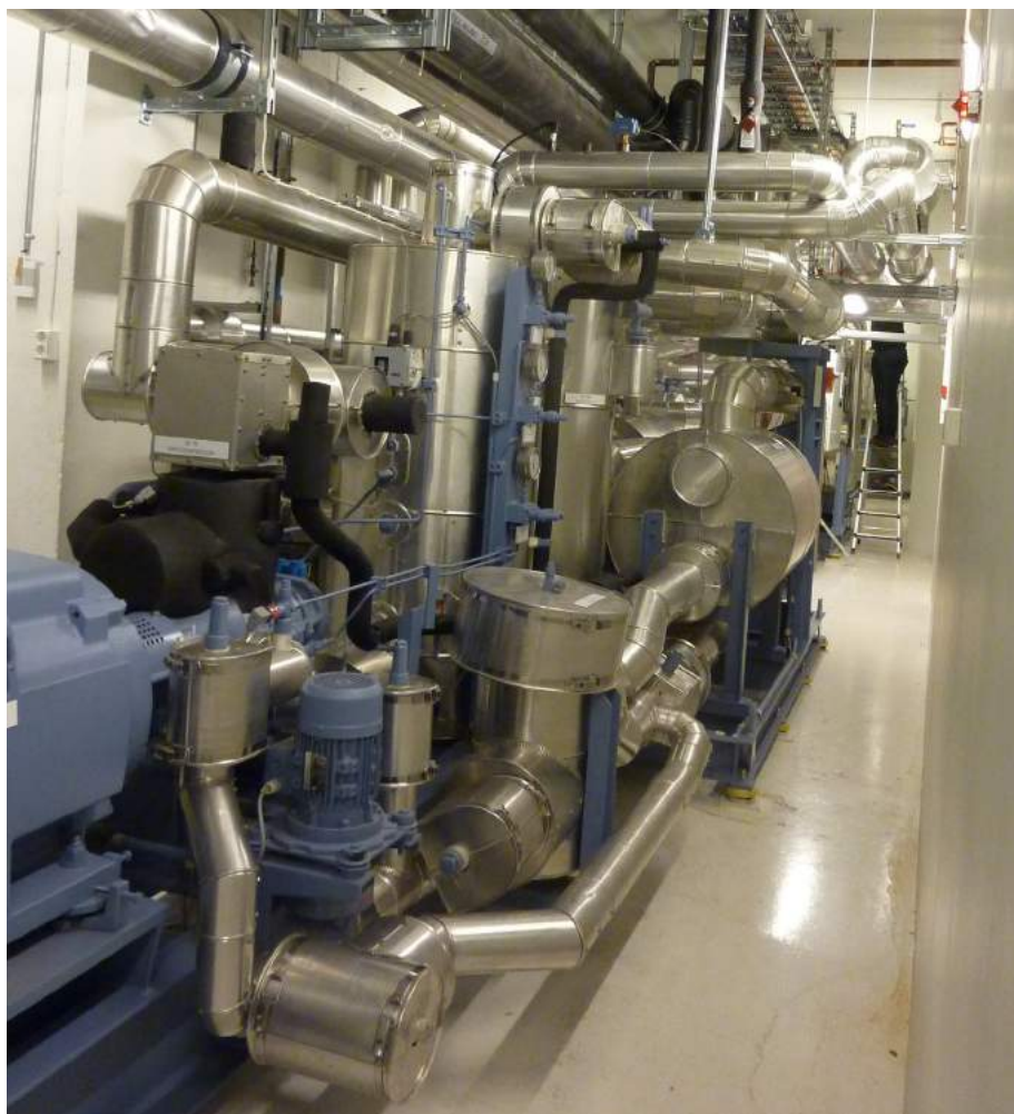
Figure 3. High-temperature liquid chiller and heat pump unit with variable speed drive twin-row compressor [Photo: Eptec Energi AS]
