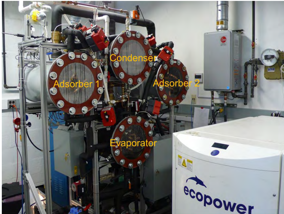
Figure 11: Photograph of combined cooling, heating and power system at UMD
