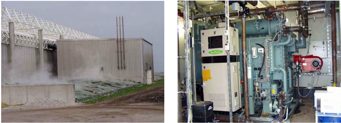
Figure 1 left: Composting hall, which is used as heat source, the machine hall where the low temperature heat is exchanged from the air to the water of the evaporator circuit and the bio filter in the front of the photo, right: the absorption heat pump
