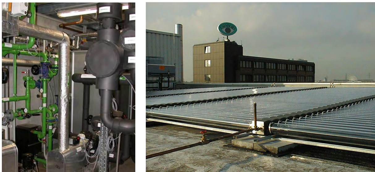
Figure 2: Solar Cooling demonstration plant at Fraunhofer UMSICHT with Yasaki WFC10 absorption chiller
