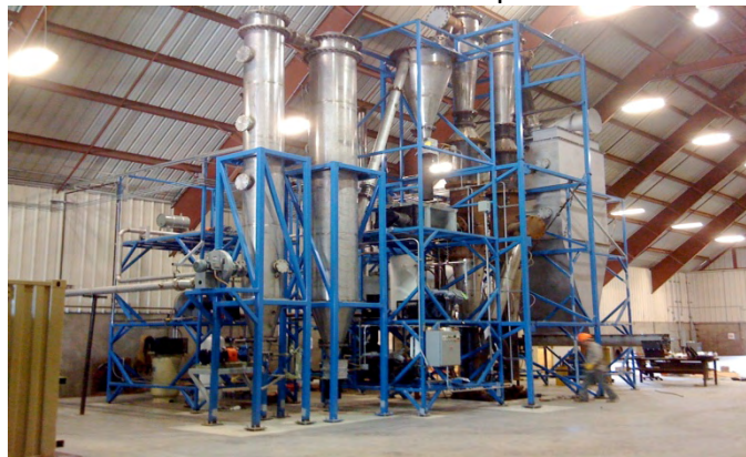
Figure: Mixed alcohols facility at University of California
